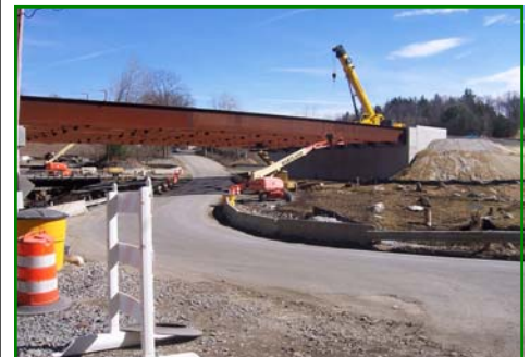
View of new Route 7 overpass at bottom of North Mountain Rd. taken on 3/8/09
